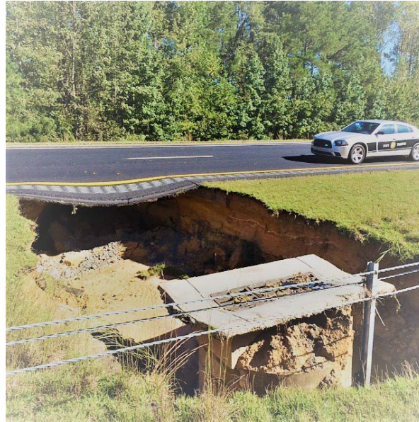
FIGURE 5.14: SINKHOLE IN NORTH CAROLINA
